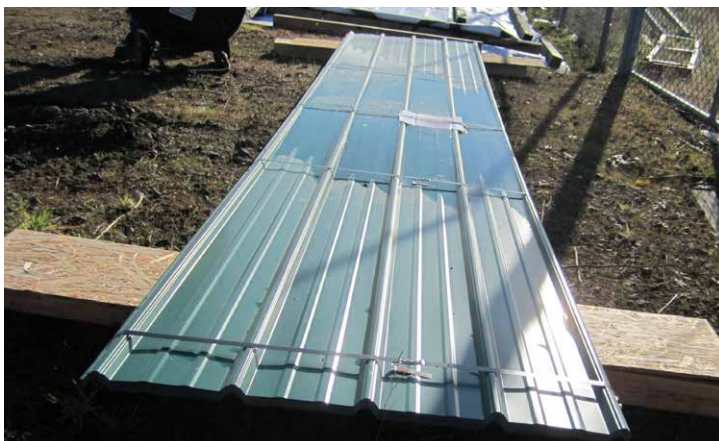
Improper Storage - Insufficient support in the center of long panels allow "Bowing" or "Sagging" that traps water in the center of the panel length.
